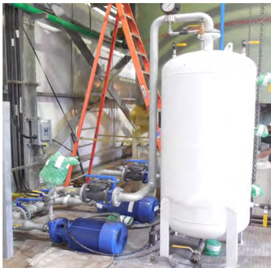
Air Pressurization Vessel and Recirculation Pumps
