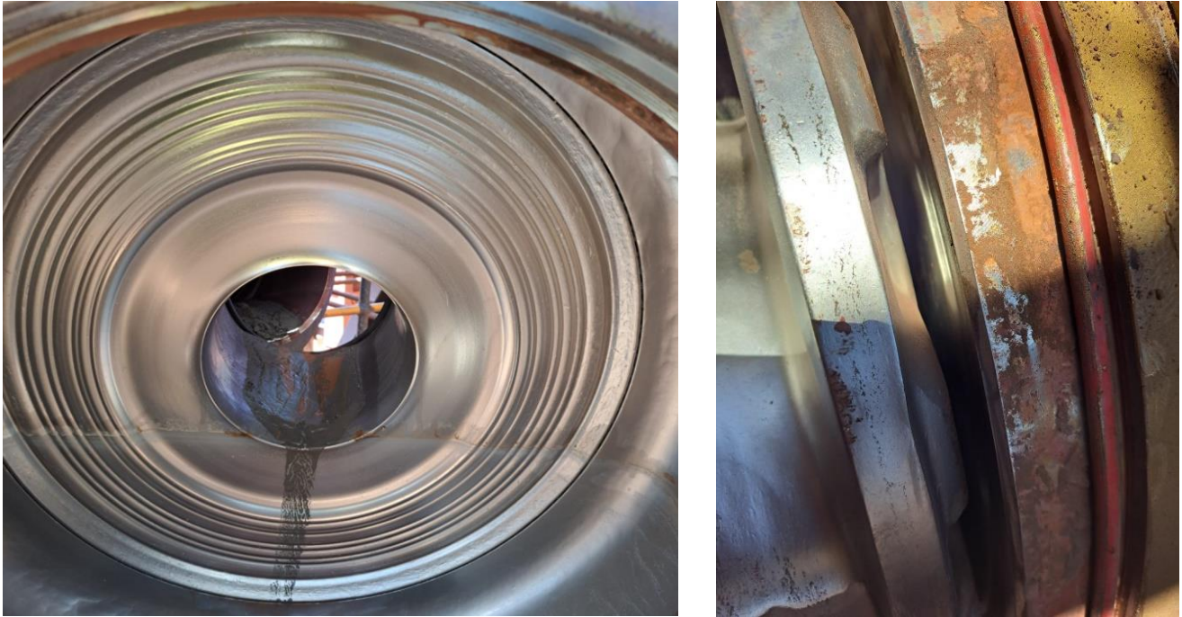
Figure 4 - Cyclone Feed Pump Suction and Drive Liner
