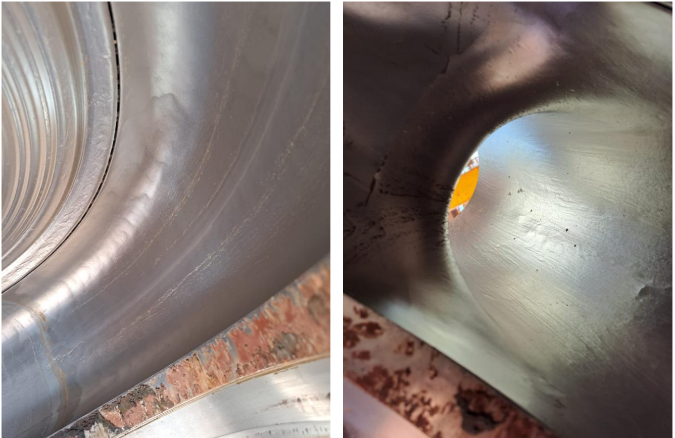
Figure 6 - Casing and Cut Water Wear
