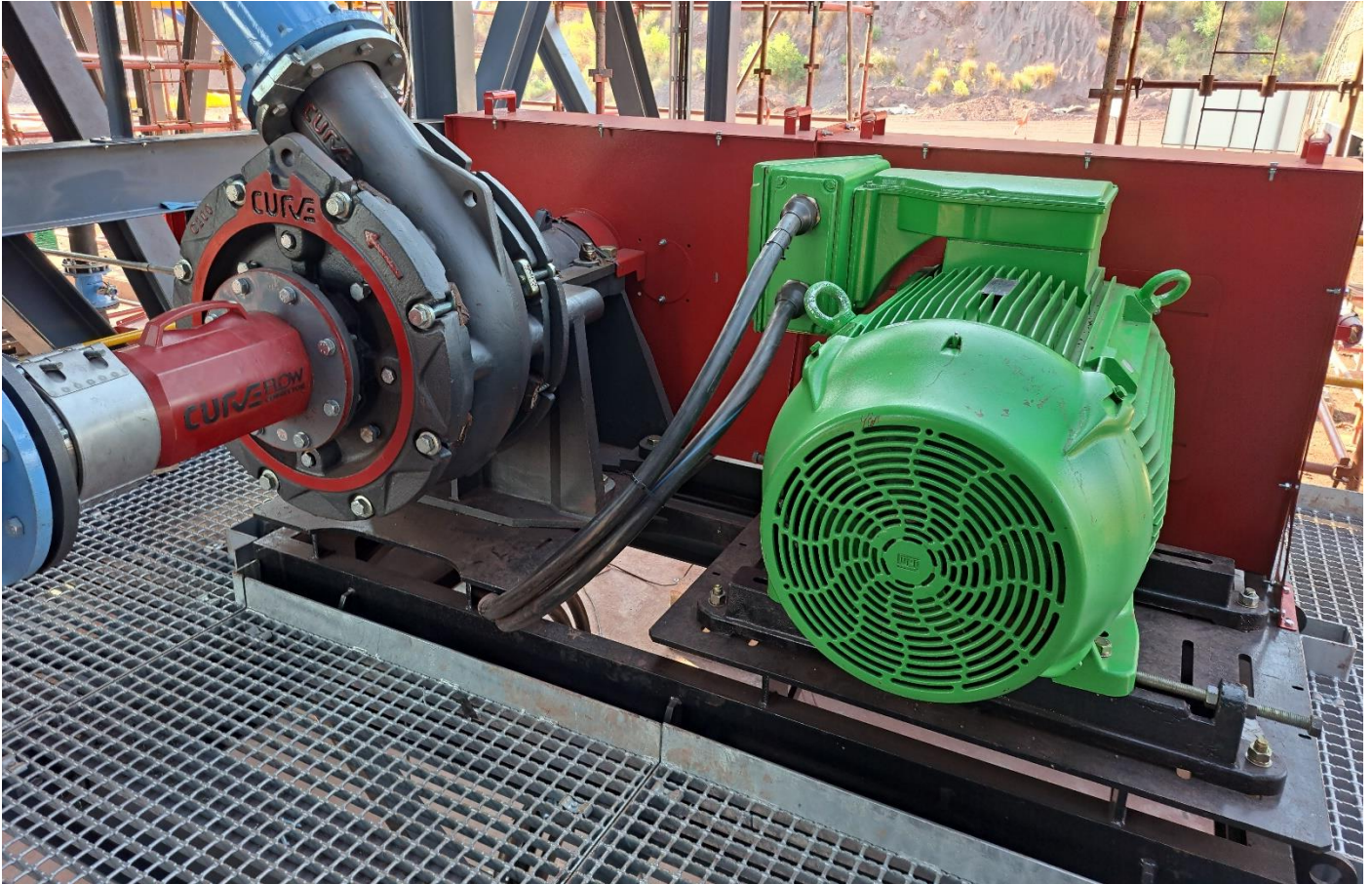
Figure 2 - Cyclone Feed Pump
